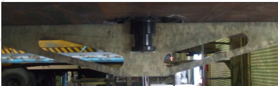
This is an example of a near perfect installation.
